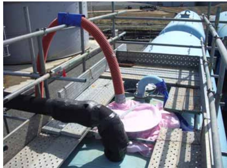
Temporary line – H2 area tank
