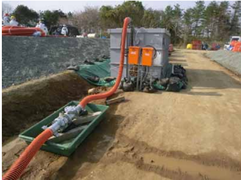
Relay tank – temporary line
