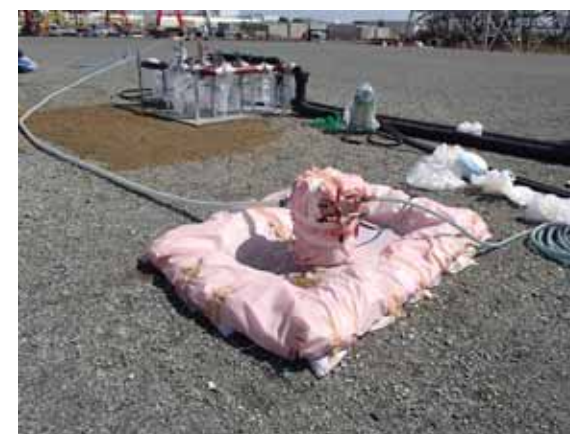
Installation of the pump at underground reservoir No. iii (photo taken on April 13)
