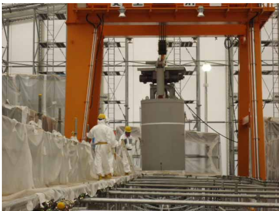
Multi-nuclide removal equipment area
