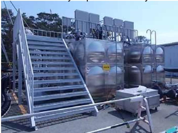
Appearance of the Standby Liquid Control System Tank (From left, Standby Liquid Control System Tank A and B)
