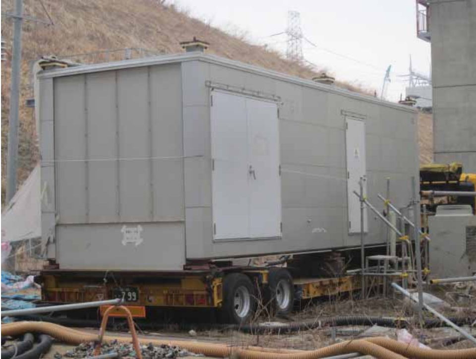
Side surface of the container, entrance of Units 3-4 temporary M/C
