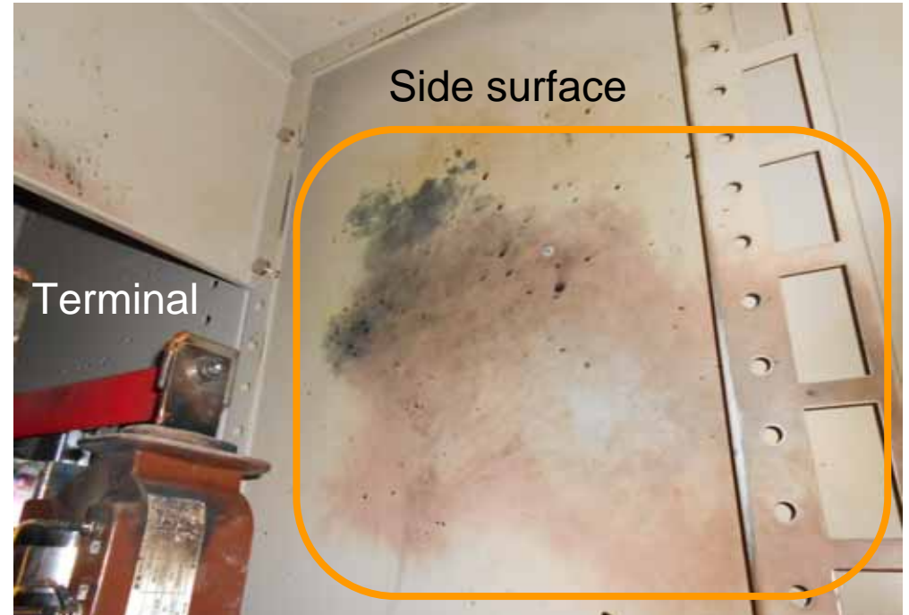
Trace of an arc found on the side surface of unit 5A
