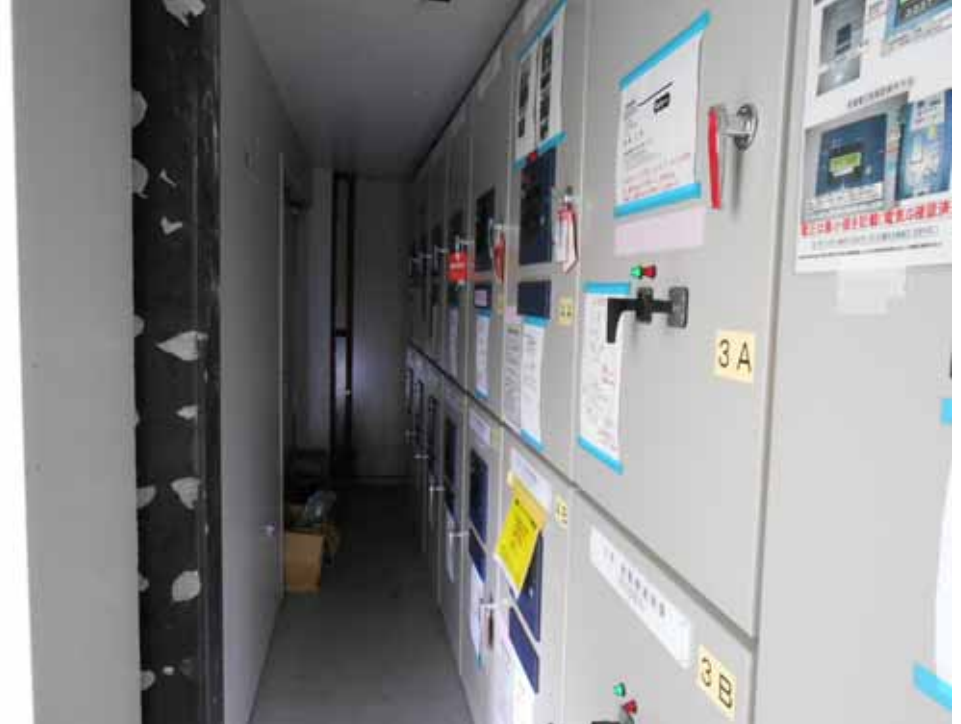
Front of Units 3-4 temporary M/C (inside the container)
