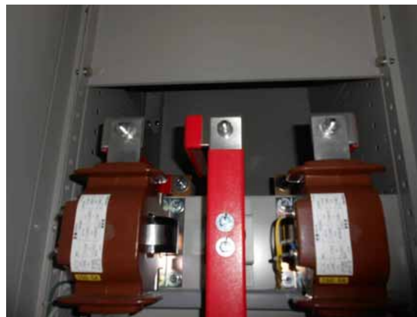
Photo 2: Sound condition of power panel
