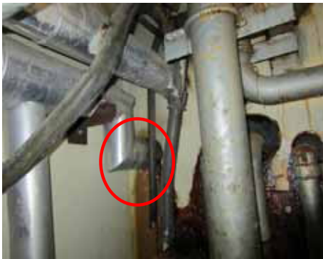
Pipe penetration area where water inflow was found
