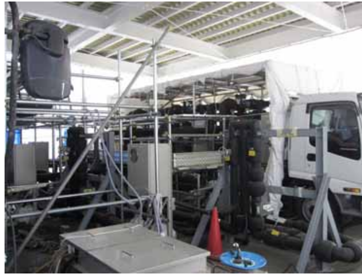
<Emergency Reactor Injection Pump on the Hill>
