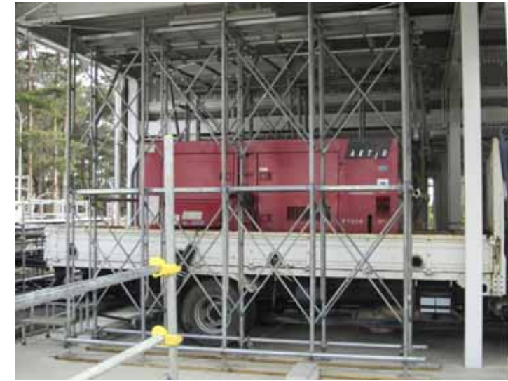
<Emergency diesel generator>
