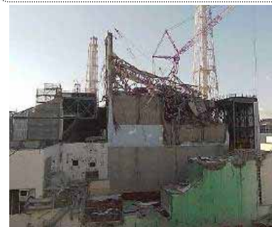
Unit 3 Reactor Building (January 29)
