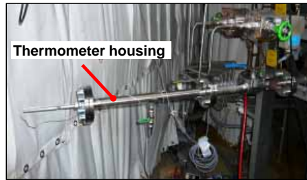
RPV Thermometer Installation Condition (October 3, 2012)
