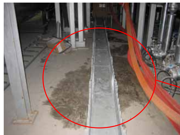
Puddle on the first floor (Photo taken on February 23 by TEPCO)
