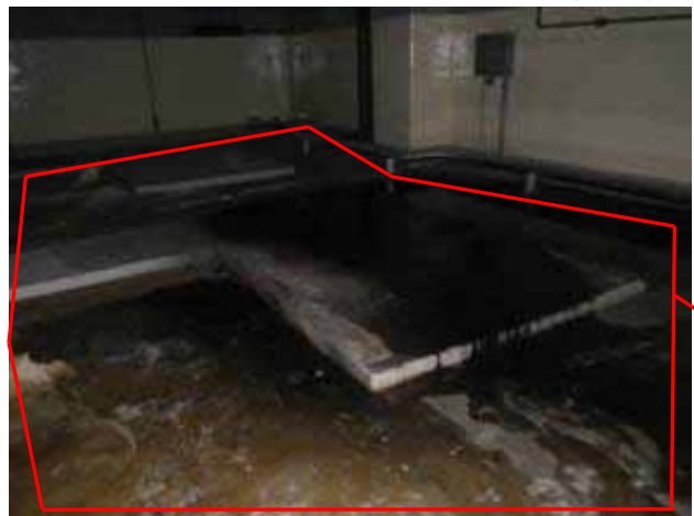
Puddle on the second floor (Photo taken on February 25 by TEPCO)
