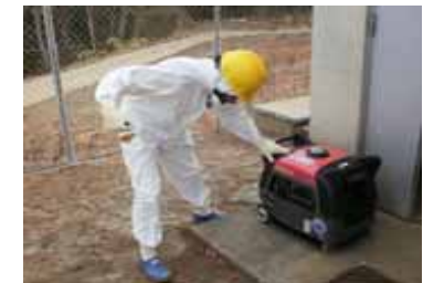
Starting the generator
