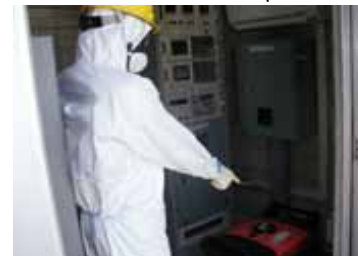
Preparation before starting the generator
