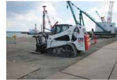
Debris removal at the site (in front of the shallow draft quay)
