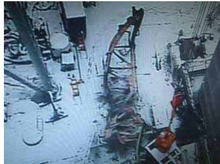
Steel truss debris (after removed)
