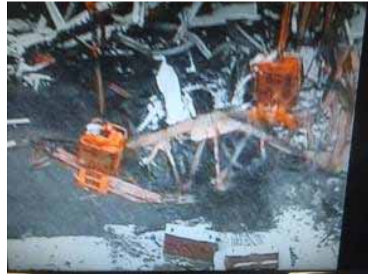
Steel truss debris (being lifted up)
