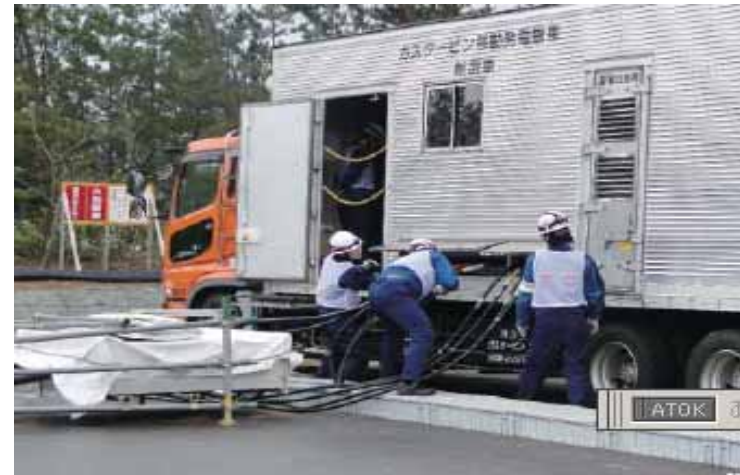
Air-cooled and on-board Gas Turbine Generator (4500kVA)
