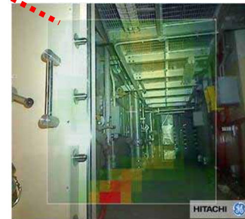
Survey on radiation source and dose rate inside the Unit 1 R/B (photo by gamma camera) (May 14~18, 2012)
