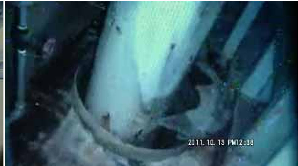
Situation of the penetration on 1 st floor with no steam release (photo as at Oct. 13, 2011)
