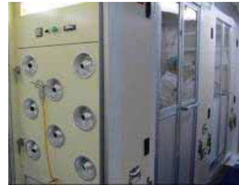
Air shower in rest place
