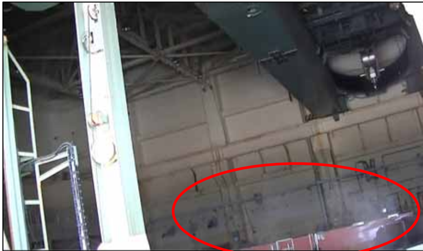
Steam release from right above the reactor on 5 th floor (photo as of Sep. 17, 2011)
