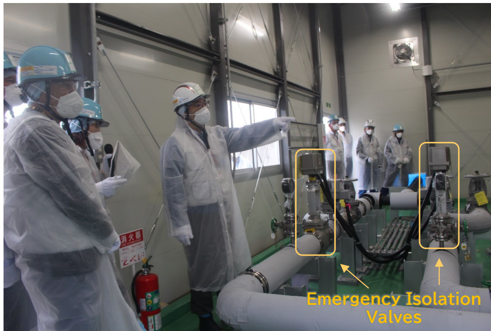
Inspection of emergency isolation valves by the International Atomic Energy Agency (IAEA) [photo taken on June 2, 2023]
