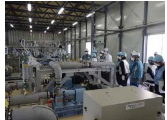
The IAEA delegation being shown the ALPS treated water transfer facility
