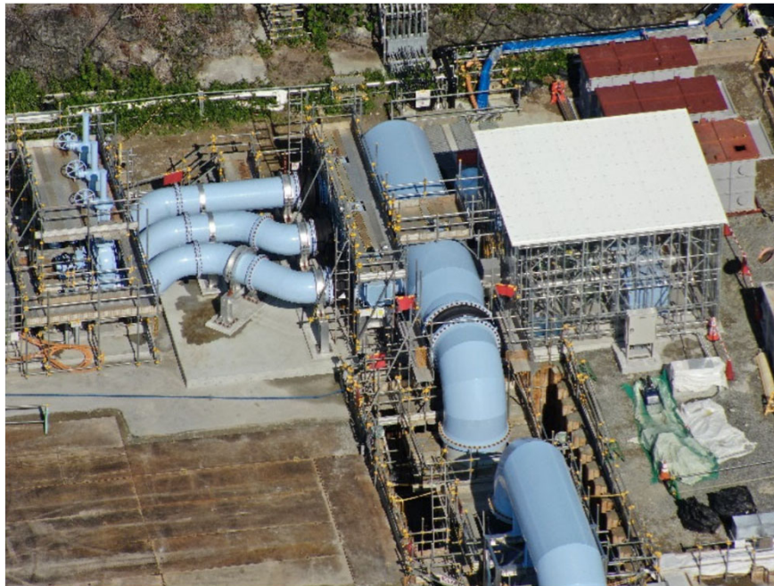
Seawater transfer pipes and seawater header pipe (Header pipe: ALPS treated water is mixed and diluted with seawater) [photo taken on June 25, 2023]
