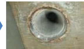
Penetration inside metal box
