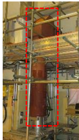
Pipe wrapped with fire retardant material
