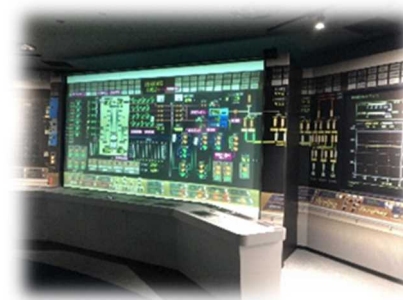
Display of main control room at Eco-ron Forest
