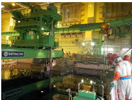
Fuel cleaning (Unit 7)
