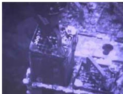
Removing fuel from the spent fuel pools
