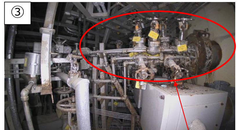
Recirculation pump instrument line
