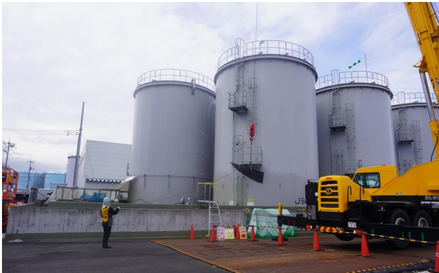
<The bottom plate was hoisted by a crane > (Photographed at around 8 AM on March 4)
