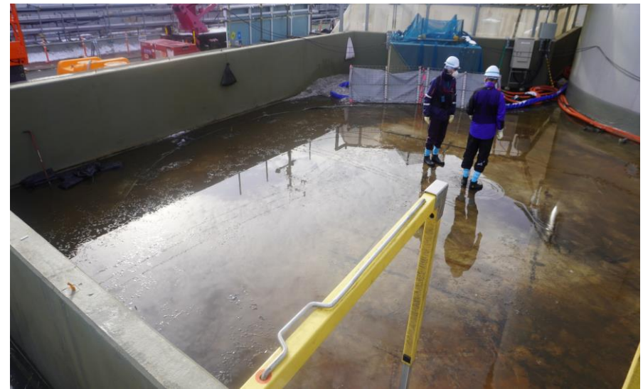
<After removal of the first tank in J9 area > (Photographed at around 8:10 AM on March 4)
