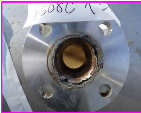
Vent pipe flange (prior to replacement)
