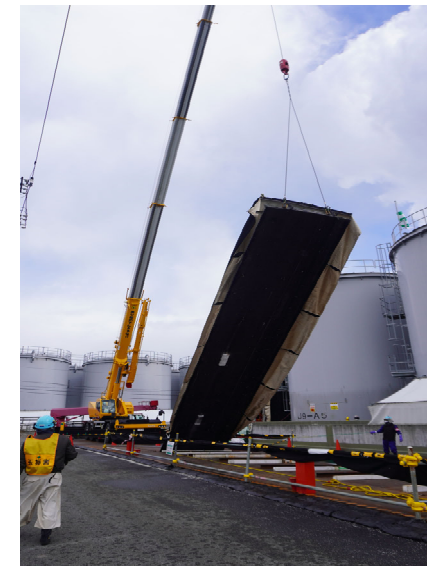
<Lowering the side plates from a tank in the J9 area to the ground > (Photographed at around 2:10 PM on February 20)
