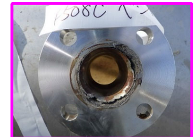
Vent pipe flange corrosion
