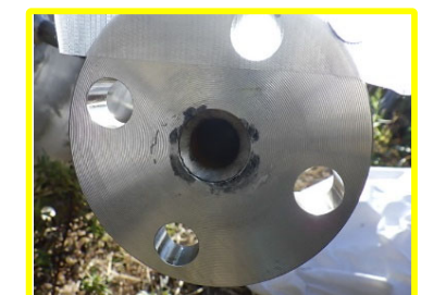
Instrument pipe flange corrosion
