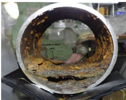
Deposits inside the pipe (Sample B)
