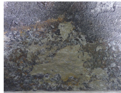
Corrosion inside the pipe (Sample D)
