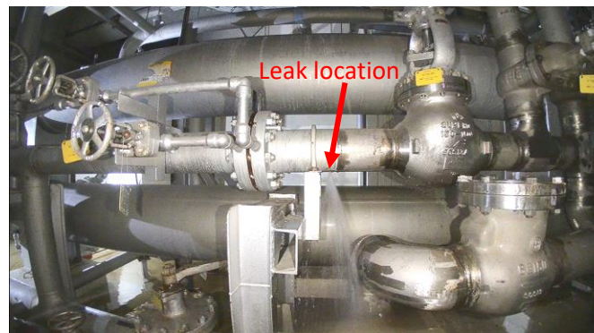
FPC heat exchanger room pipe conditions (photographed with a drone on October 1) *The water leak was stopped after the investigation
