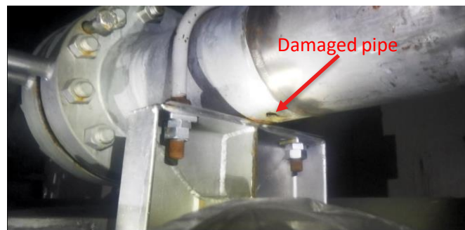
FPC heat exchanger room pipe conditions (photographed by a worker on October 2)
