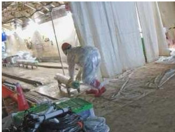
Transporting at the push pipes from the large freight loading entrance on the first floor of the reactor building to the west passageway
