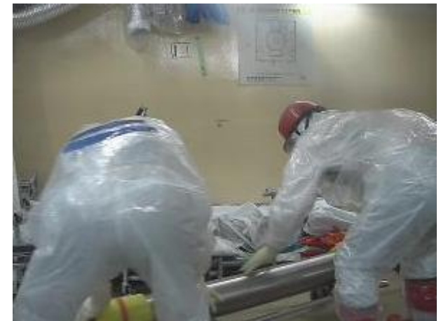
Transporting the push pipe from the west passageway on the first floor of the reactor building
