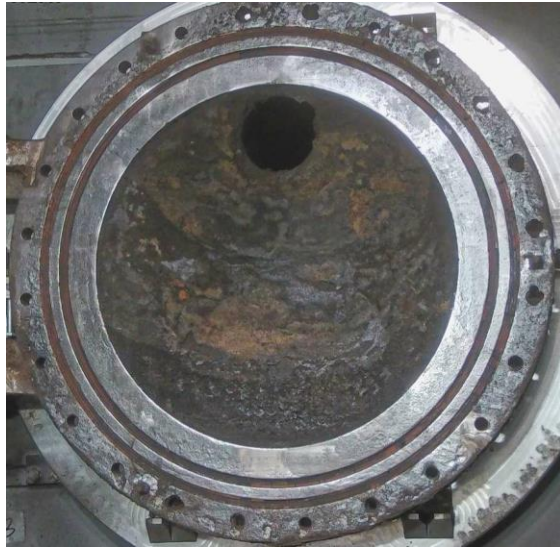
X-6 penetration (before the removal of deposits)
