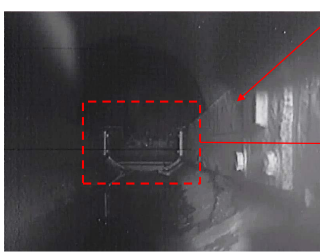
Condition of the X-6 penetration after the deposit removal (from the front to the back)
