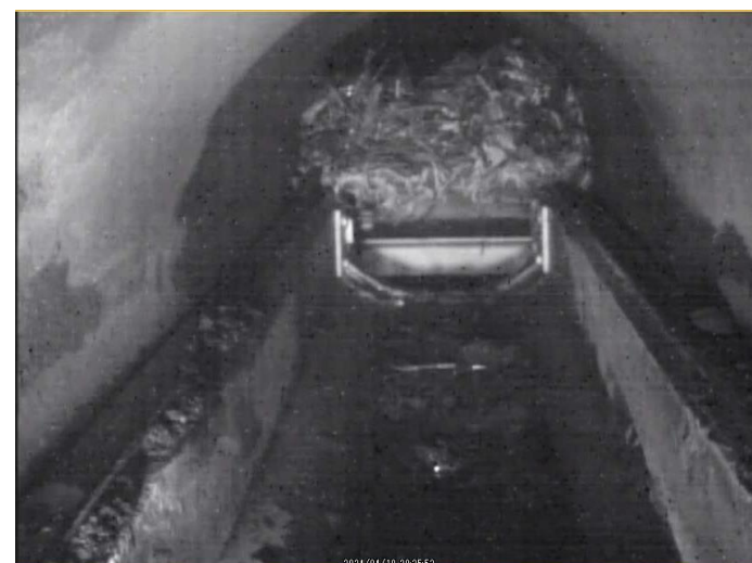
After removal of the cables at the bottom of the X-6 penetration
