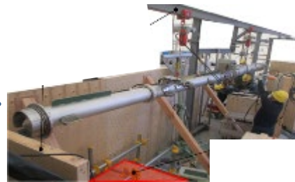
Spray jig installation ※Connected to X-53 penetration
