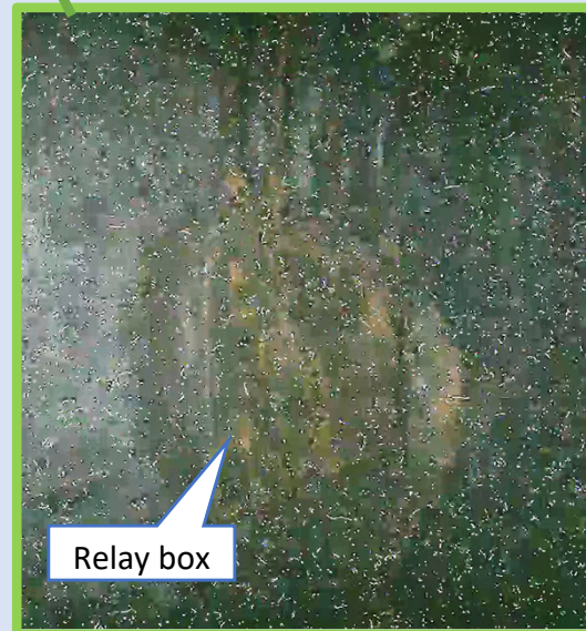
Condition of relay box inside the pedestal (left: around 0°, right: around 180°)
