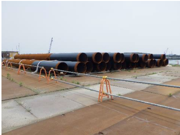
Figure 3. Steel pipe piles that were used (temporarily stored on site) (Photo taken on June 8, 2023)
