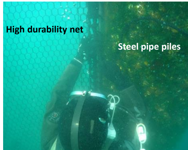
Figure 7. Divers attaching the high durability net to the steel pipe piles (Photo taken on January 13, 2024)
