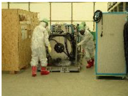
Installation of deposit removal equipment (high pressure water, abrasive water jet)
