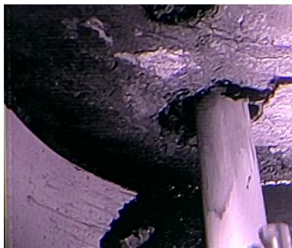
Deposit collapse caused by pushing with the dozer rod on the bottom left side of X-6 penetration (photo taken on January 11)
