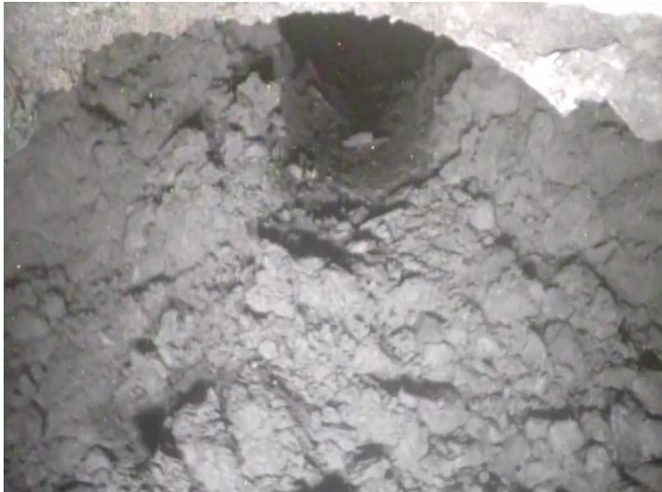
Before the work of low pressure water (top of X-6 penetration) (photo taken on January 16)
