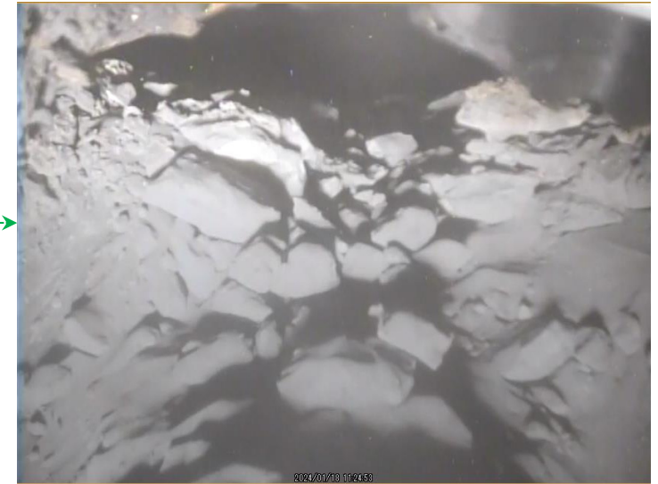
After the work of low pressure water (top of X-6 penetration) (photo taken on January 18)
