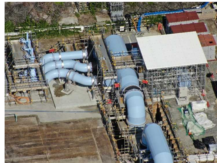
Building the seawater transfer pipe foundation and installing the seawater pipe header
