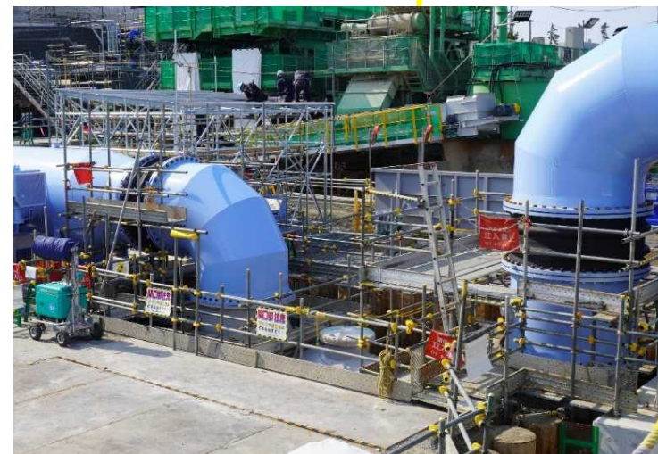
Building the seawater transfer pipe foundation and installing the seawater pipe header
