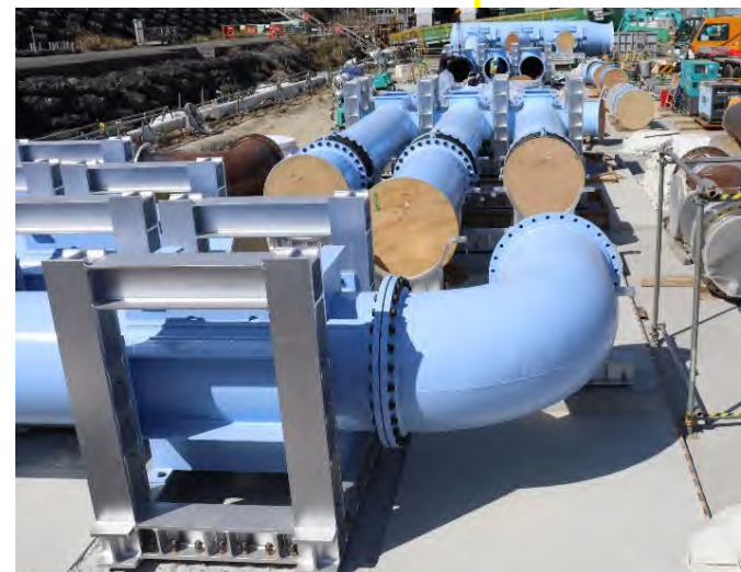
Building the seawater transfer pipes foundation and installing the seawater pipe header
