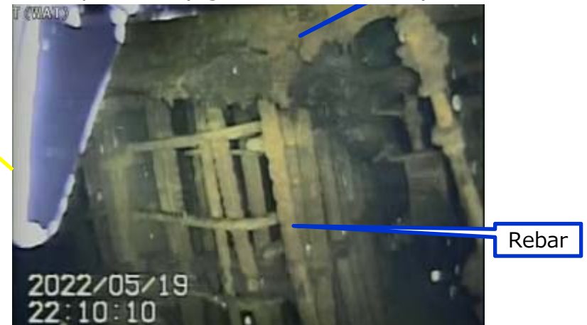
Photo 3. Conditions at the bottom of the deposits at the pedestal opening (right side foundation)
