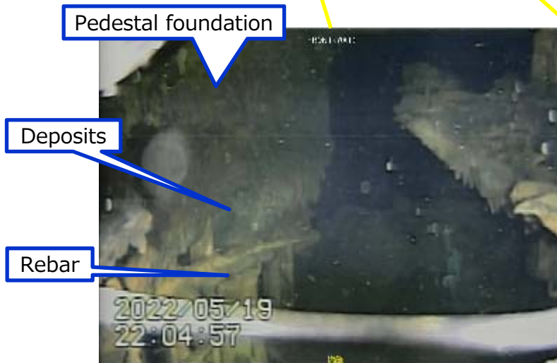
Photo 2. Conditions above and below the deposits at the pedestal opening (left side foundation)
