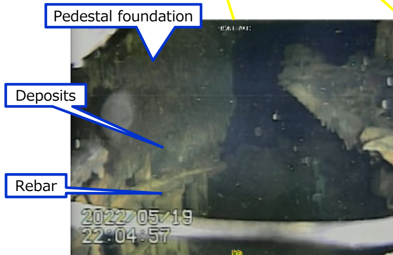
Photo 2. Conditions above and below the deposits at the pedestal opening (left side foundation)
