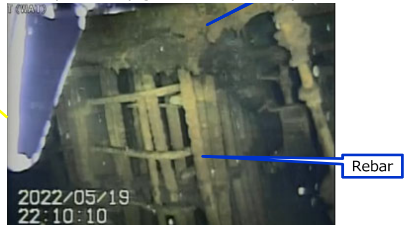
Photo 3. Conditions at the bottom of the deposits at the pedestal opening (right side foundation)
