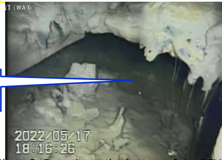
Photo 3. Deposits at the bottom of the PCV (hollow area)
