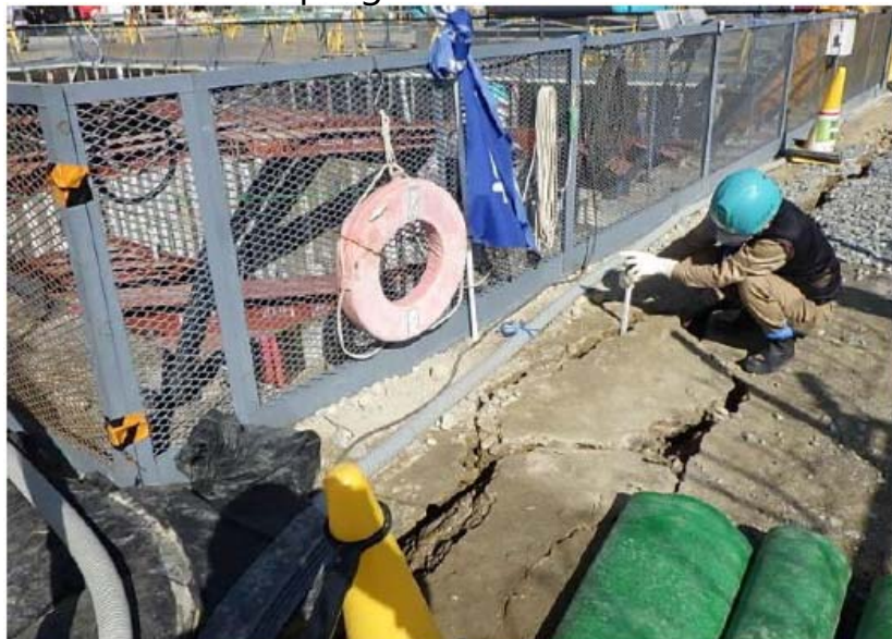
Photo ① Cracks on the ground after the earthquake (near the downstream storage)
