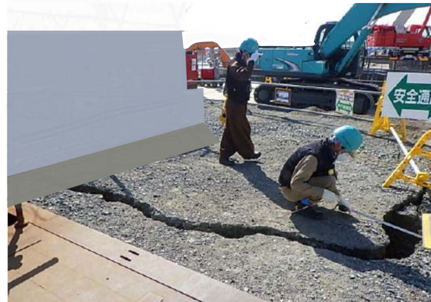
Photo ② Cracks on the ground after the earthquake (around the downstream storage)
