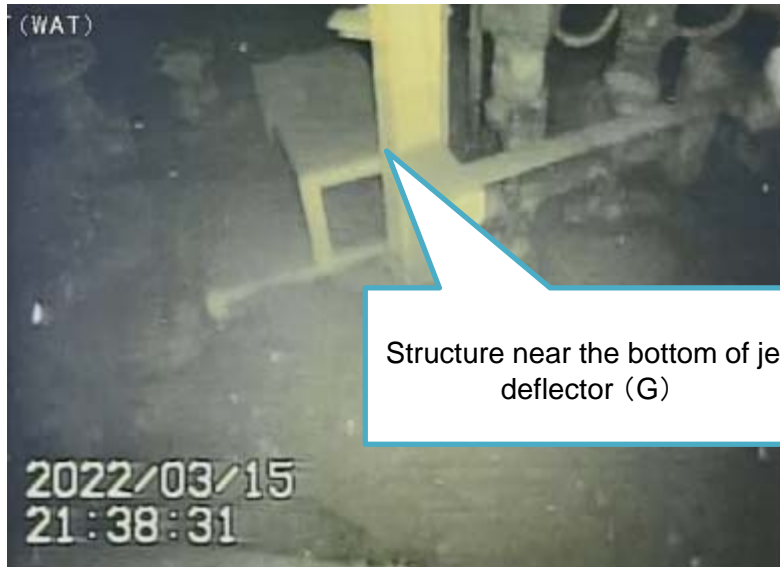
Photo 2. Conditions near the bottom of jet deflector (G)①
