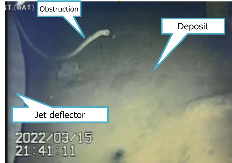
Photo 3. Conditions near the bottom of jet deflector (G) ② 8
