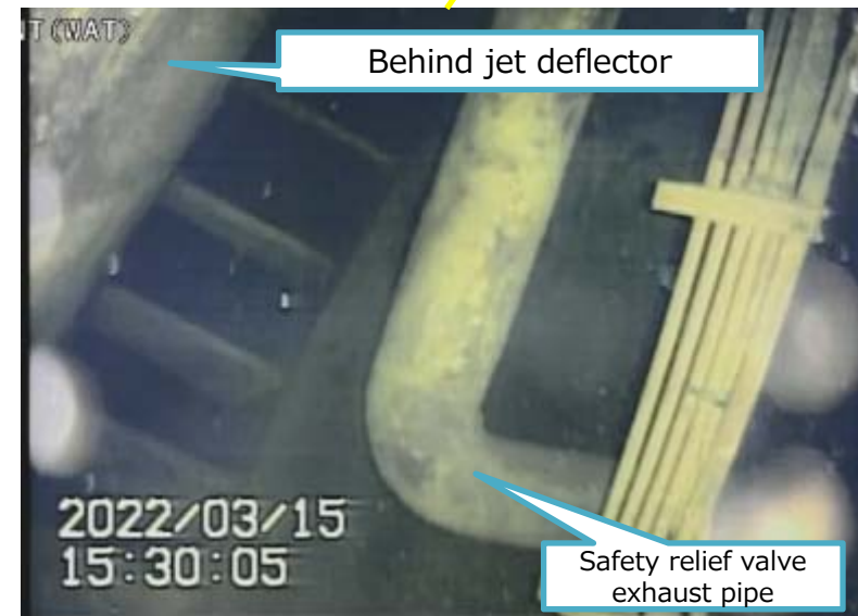
Photo 3. Conditions behind jet deflector (G)
