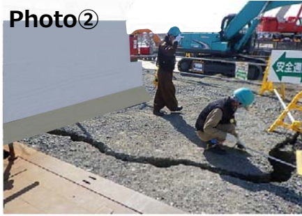
Surface cracks/ground subsidence
