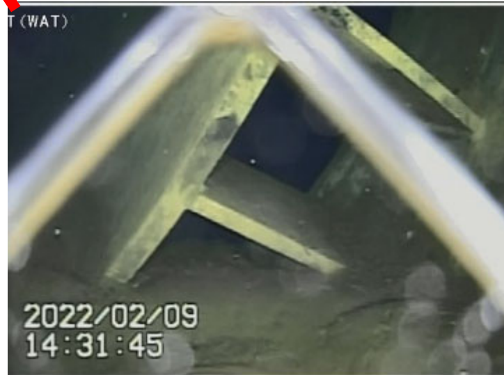
Conditions to the east-northeast of the PCV (close-up)
