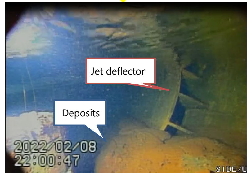
Deposits near the 4 th jet deflector
