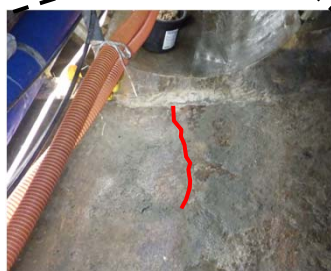
Crack (Length: Approx. 1.0m, Width: Approx. 5.0mm)
