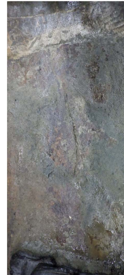
Enlarged photo of crack
