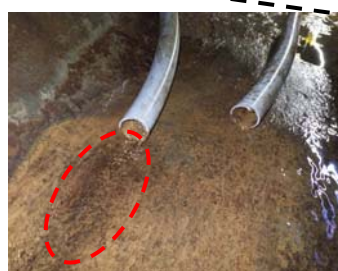
Spring water location (Water conveyance pipe)
