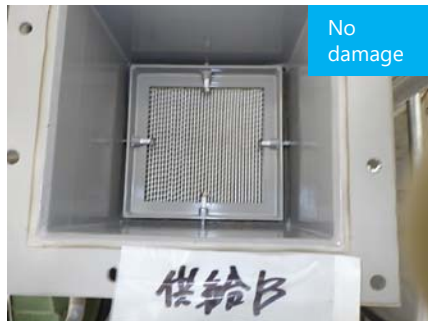
Existing ALPS feed tank B
