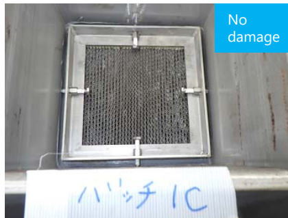
Existing ALPS batch treatment tank 1C
