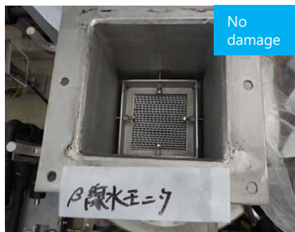
Existing ALPS β ray water monitor sample temporary reception tank
