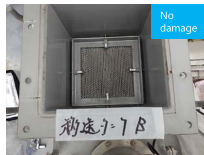
Existing ALPS transfer tank B
