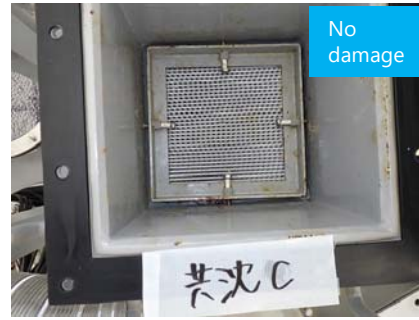
Existing ALPS coprecipitate tank C
