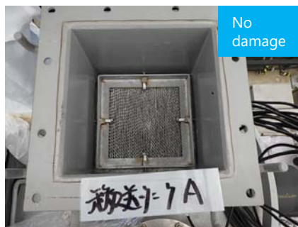
Existing ALPS transfer tank A
