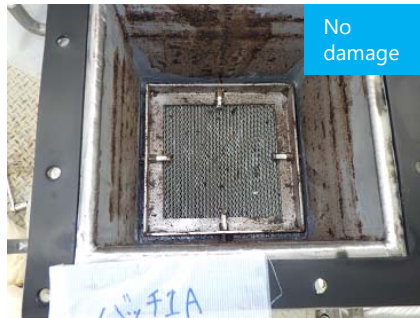
Existing ALPS batch treatment tank 1A
