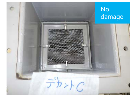
Existing ALPS decanting tank C
