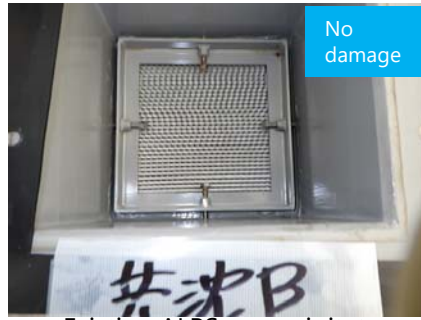
Existing ALPS coprecipitate tank B
