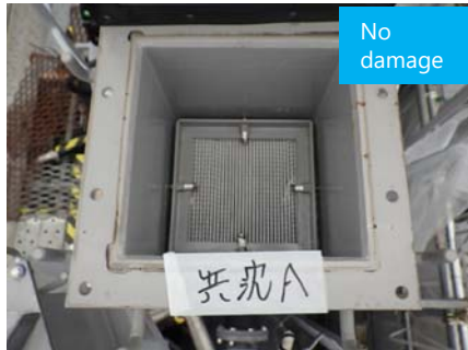
Existing ALPS coprecipitate tank A
