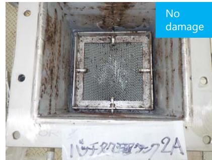
Existing ALPS batch treatment tank 2A
