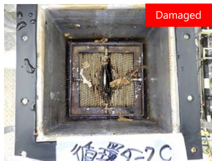
Existing ALPS circulation tank C
