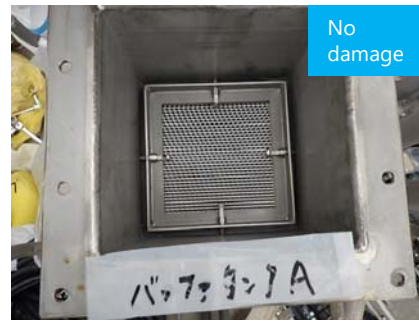
Existing ALPS buffer tank A
