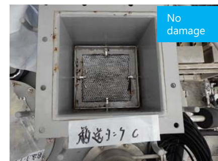
Existing ALPS transfer tank C
