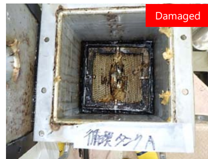
Existing ALPS circulation tank A
