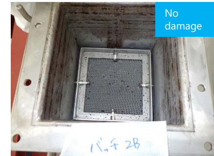
Existing ALPS batch treatment tank 2B
