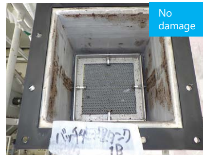
Existing ALPS batch treatment tank 1B
