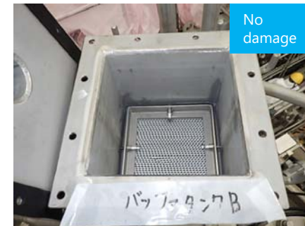
Existing ALPS buffer tank B
