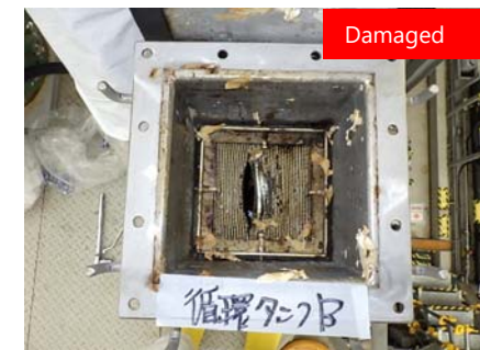
Existing ALPS circulation tank B
