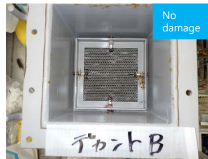
Existing ALPS decanting tank B
