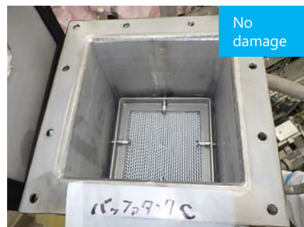
Existing ALPS buffer tank C
