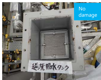
Existing ALPS backwashing water tank
