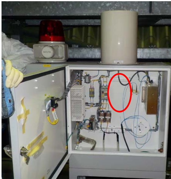
①Area radiation monitor detector box (Photograph taken prior to the earthquake, the aforementioned fuse is located in the area of the red circle)
