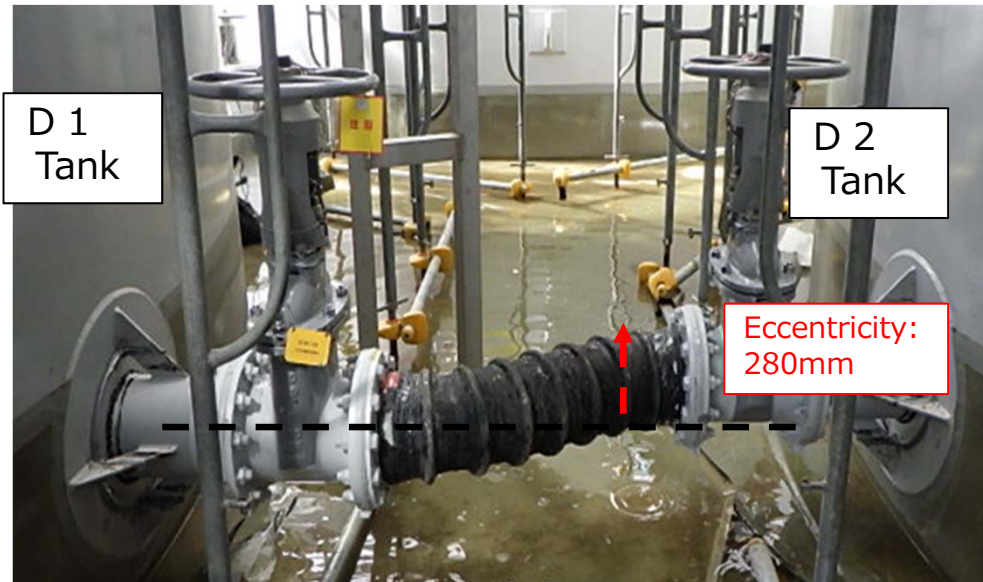
Coupling pipe (Connecting D1-D2) (A small amount of rain water has accumulated inside the dyke)
