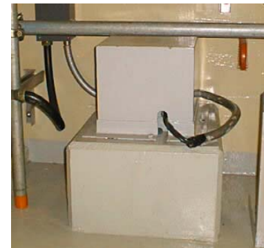
(Reference) Permanent seismometer in Unit 6
