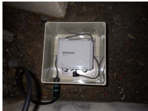
Simple seismometer installed in Unit 3 on a trial basis ※ (1 st floor level)
