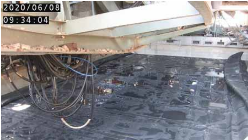
4. SFP after inserting and spreading the cover bag (Photo taken on June 8)
